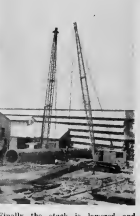
Finally the stack is lowered and moved away on a dolly. It will be used's next Acid Plant furnace up high enough so they will be carried out to sea.
